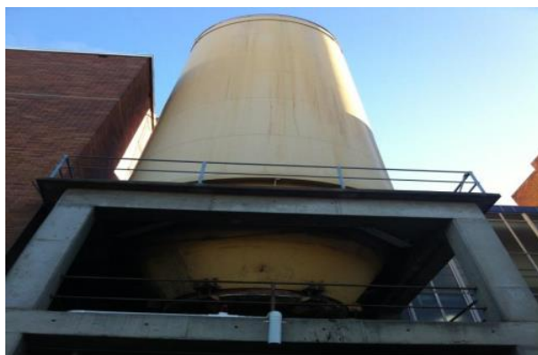
Photo 5.3.6 –Waste holding silo
