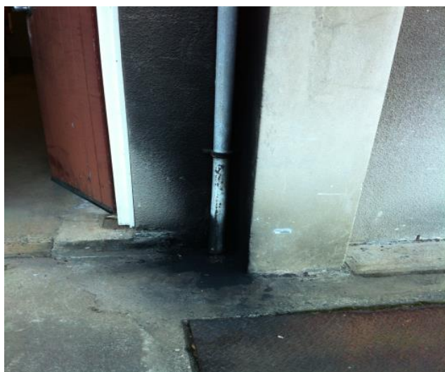
Photo 5.9.3 – Black staining of floor outside southern pump room door
