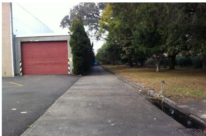
Photo 5.1.13 – View of concrete driveway to the west of the building (looking south)
