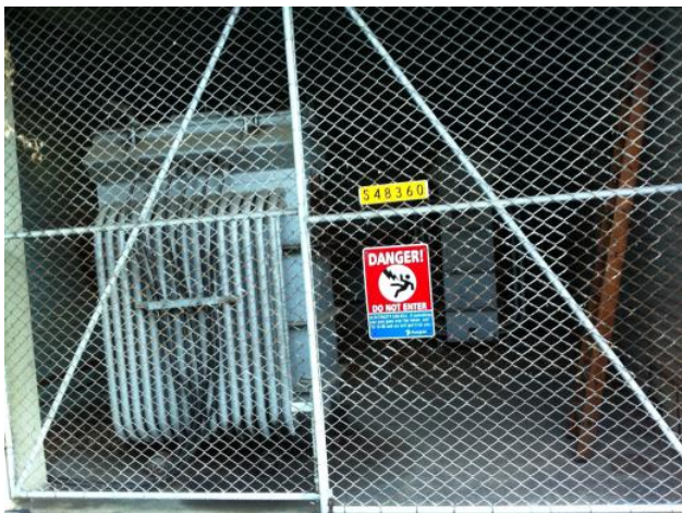
Photo 5.9.2 – View of the Transformer room and the staining of floor at the bottom
