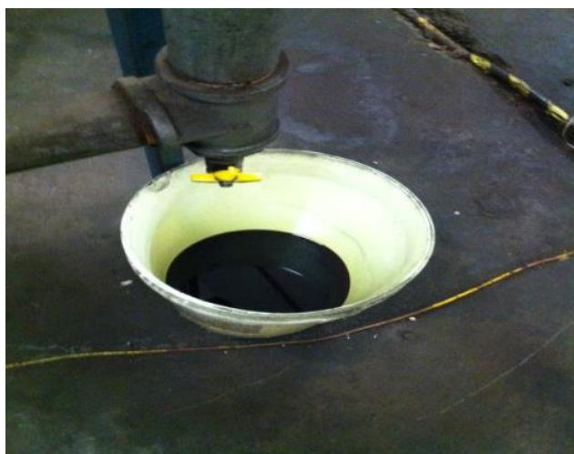
Photo 5.7.1 – Storage of leaked compressor oil in a bucket
