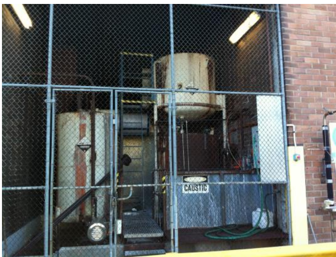
Photo 5.3.9 – Caustic soda room
