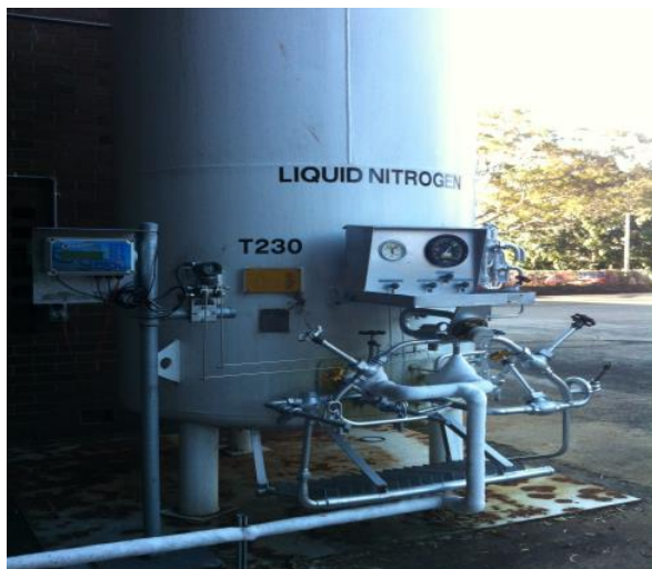
Photo 5.5.1 – Liquid nitrogen AST
