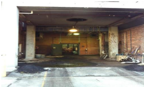
Photo 5.3.5 – Grout area and the oil-water separator room at the back. On top of the ceiling is the bottom opening of waste holding silo.
